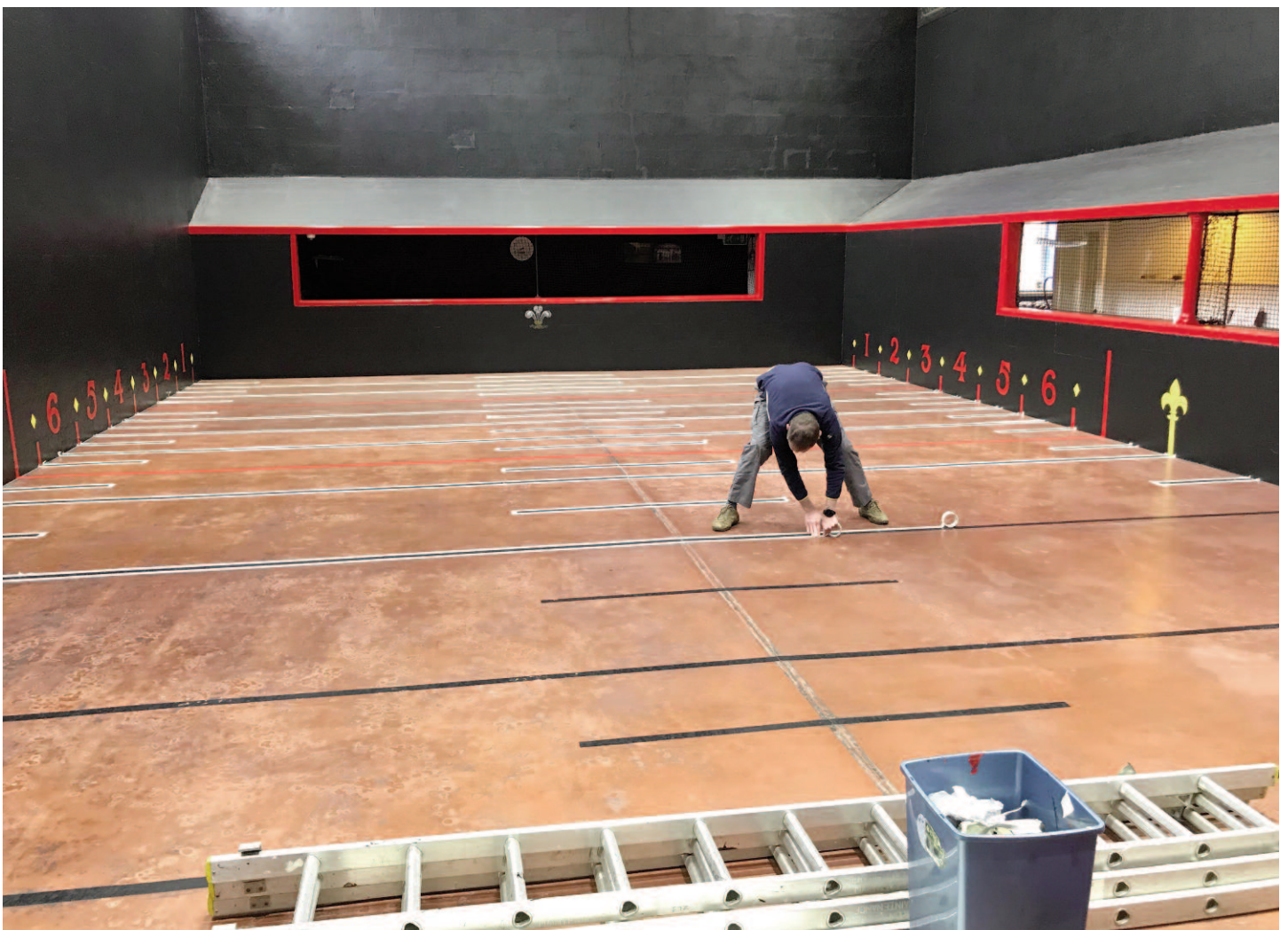
Floor complete, walls and markings, corridor and bandeau painted. Just the chase lines to do; Adam Jeffrey giving his back a good work-out!
